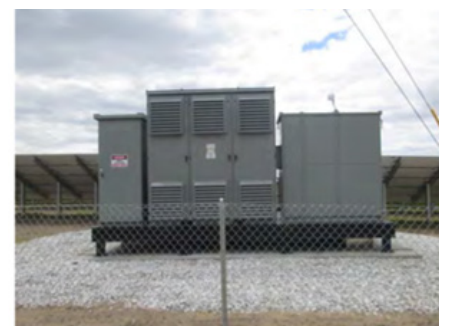
Solar Power Transformer Beardstown, IL
